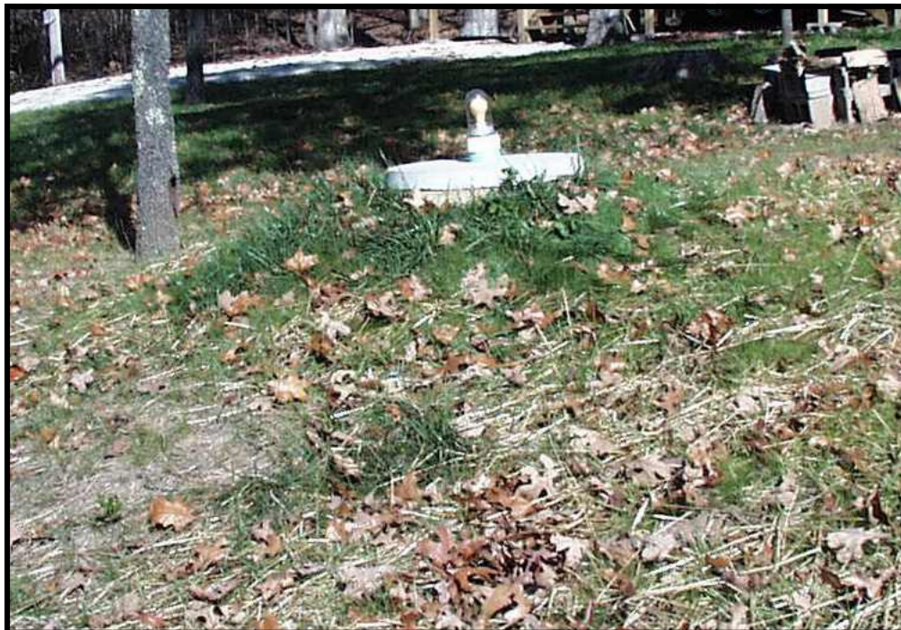
Malfunctioning Holding Tank. The bright, lush green grass around the top of the manhole cover is evidence that the holding tank has been leaking due to the lack of proper MAINTENANCE and routine pumping.
