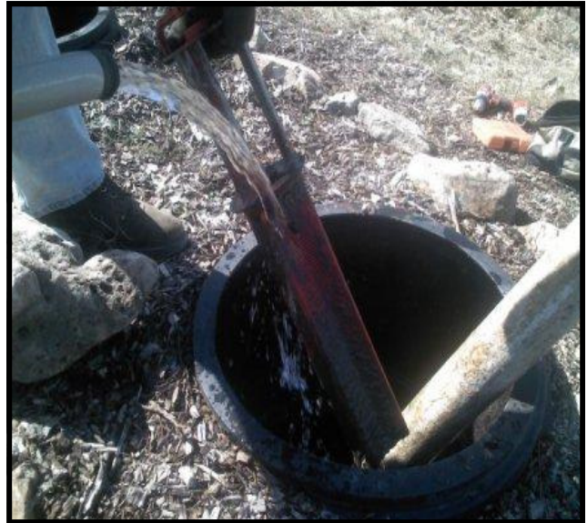
Properly cleaning a dirty effluent screen.
