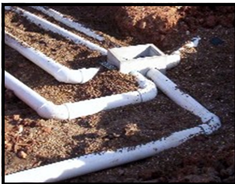
Concrete distribution box
