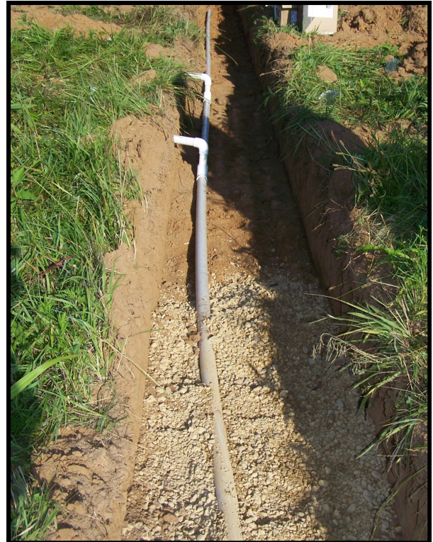
Low Pressure Pipe Manifold. The manifold trench and connections to LPP valves and distribution lines.
