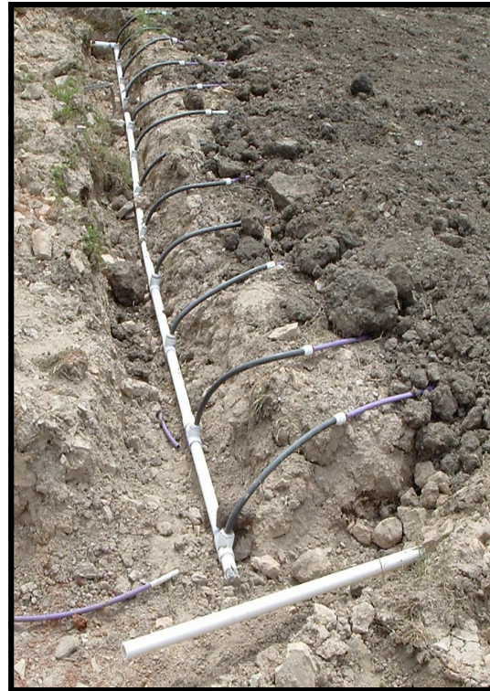
Subsurface Drip Dispersal. A manifold trench and supply manifold line is shown with flexible pipe connected to the small diameter drip irrigation lines. The return manifold from the opposite end of the zone is shown in the foreground. Drip lines are often plowed into the soil; this photo shows suitable imported soil used to cover the drip lines.
